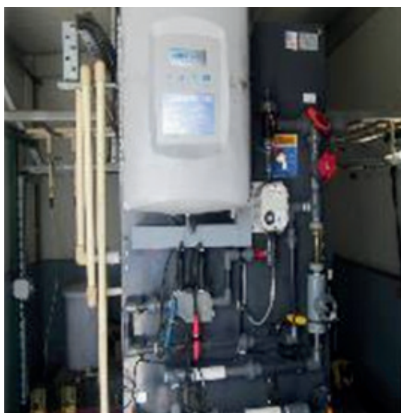
Auto blowdown system Installation & synchronization with 3D TRASAR
