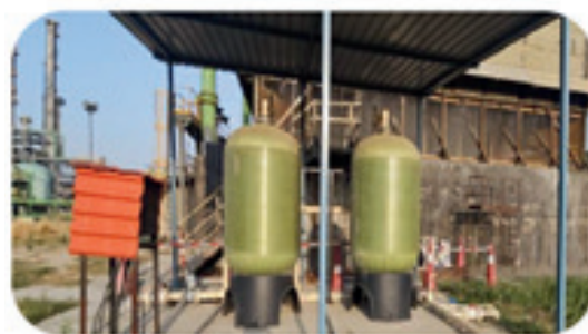
Rooftop Rainwater Treatment
