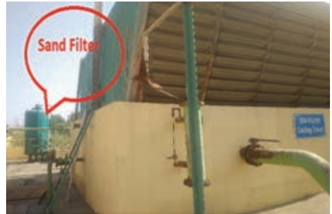
Side Stream Filter In Cooling Tower Water Circuit
