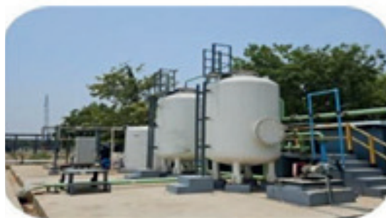
Rainwater Treatment Plant
